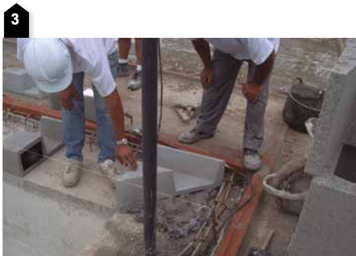
We start by positioning the pieces of the corners using a laser level. We place twine between them. Then we position the S9 blocks between corner and corner.
