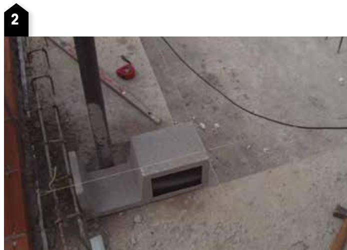
To simplify the process of concreting, this may be done in two stages. First a flat reception area is left with some reinforced iron bars and we place the hydro-expansive joint FUGA STOP MINI in the middle of the reinforced bars. Then it is finished by filling the gap (after step 5).
