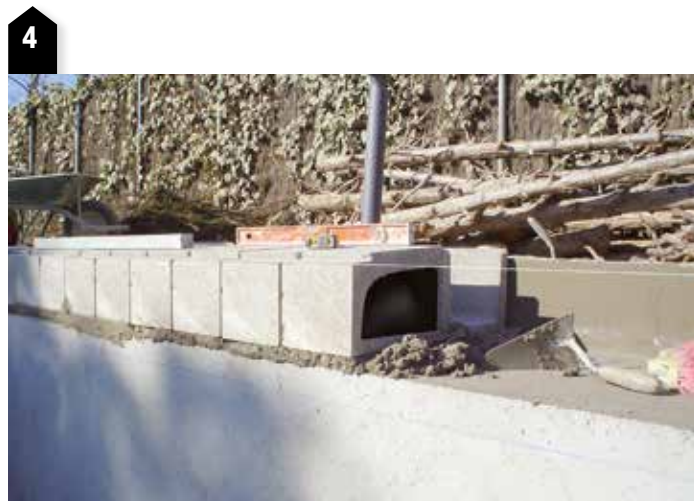
The concrete blocks are positioned with mortar to which a latex type additive such as PRIMFIX has been added with 1 part PRIMFIX to 2 parts water.
