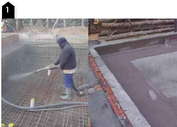
The concrete is cast, forming the walls, tank bottom and perimeter low wall, leaving a reception area for laying the S9 block according to its measurements.
